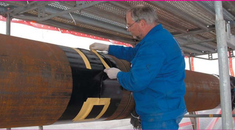
DMS-Installation am Objekt
