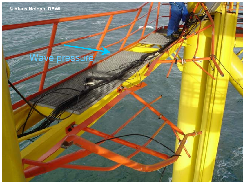
Fig.14: High orbital speeds of the extreme waves on 1.11. 2006 have torn away the railing of the 15m walkabout and destroyed 50% of the cables which connect the structural dynamic sensors to the platform main deck.
