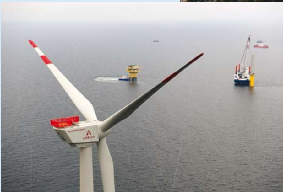
Fig. 4-6: Erection of the first wind turbine in the alpha ventus offshore test site (Source: DOTI 2009)
