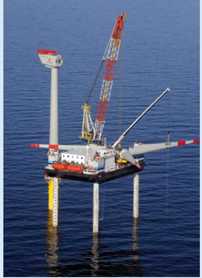
Fig. 2: Construction site alpha ventus. The rotor is attached to a wind turbine in the test site in July 2009 (Source: DOTI 2009)
